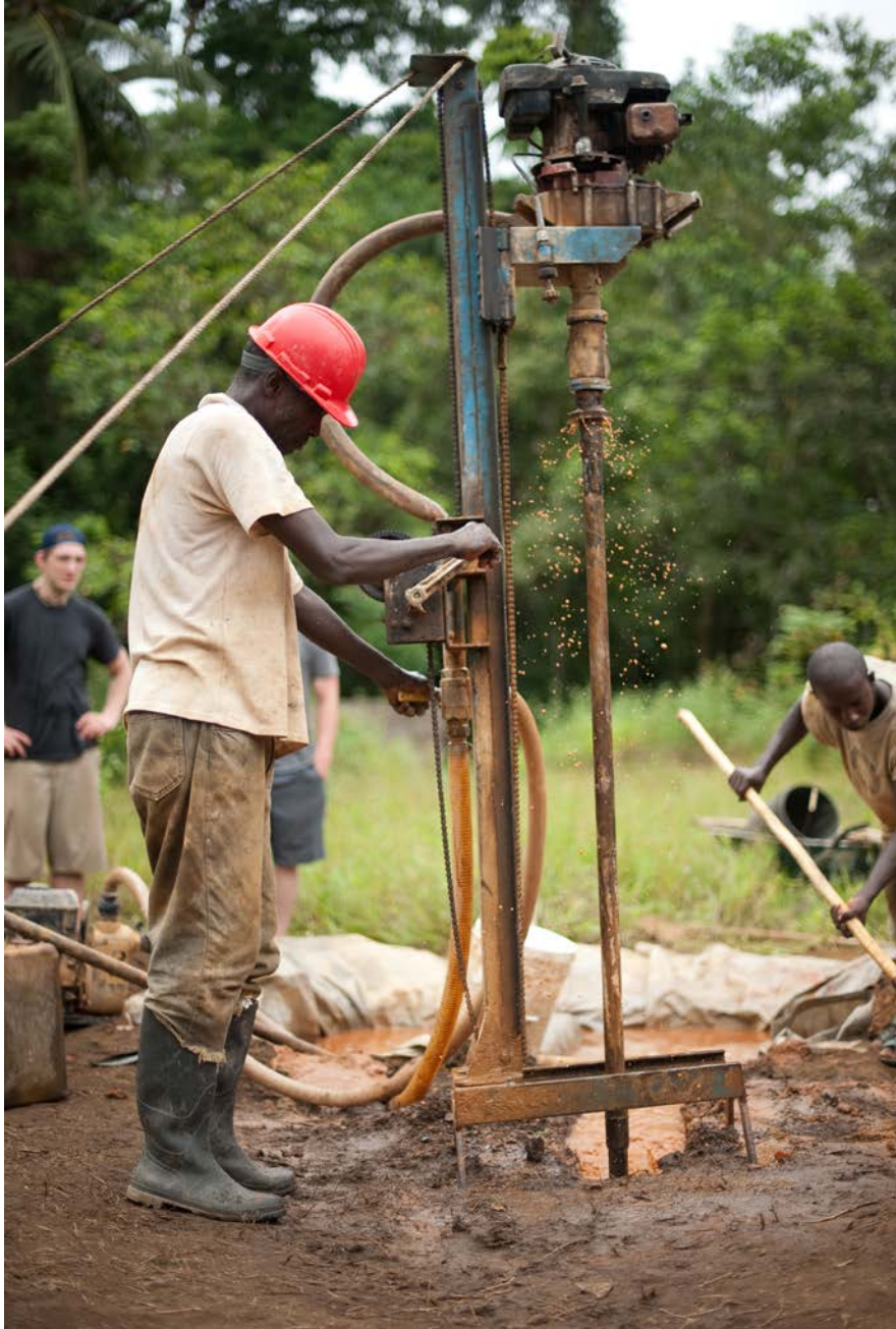
Joe Qua Qua, head driller, has nine years of experience operating the LS100 by Lone Star Drills. He and the team are drilling a well for a village near the Bensonville Highway in Liberia.
