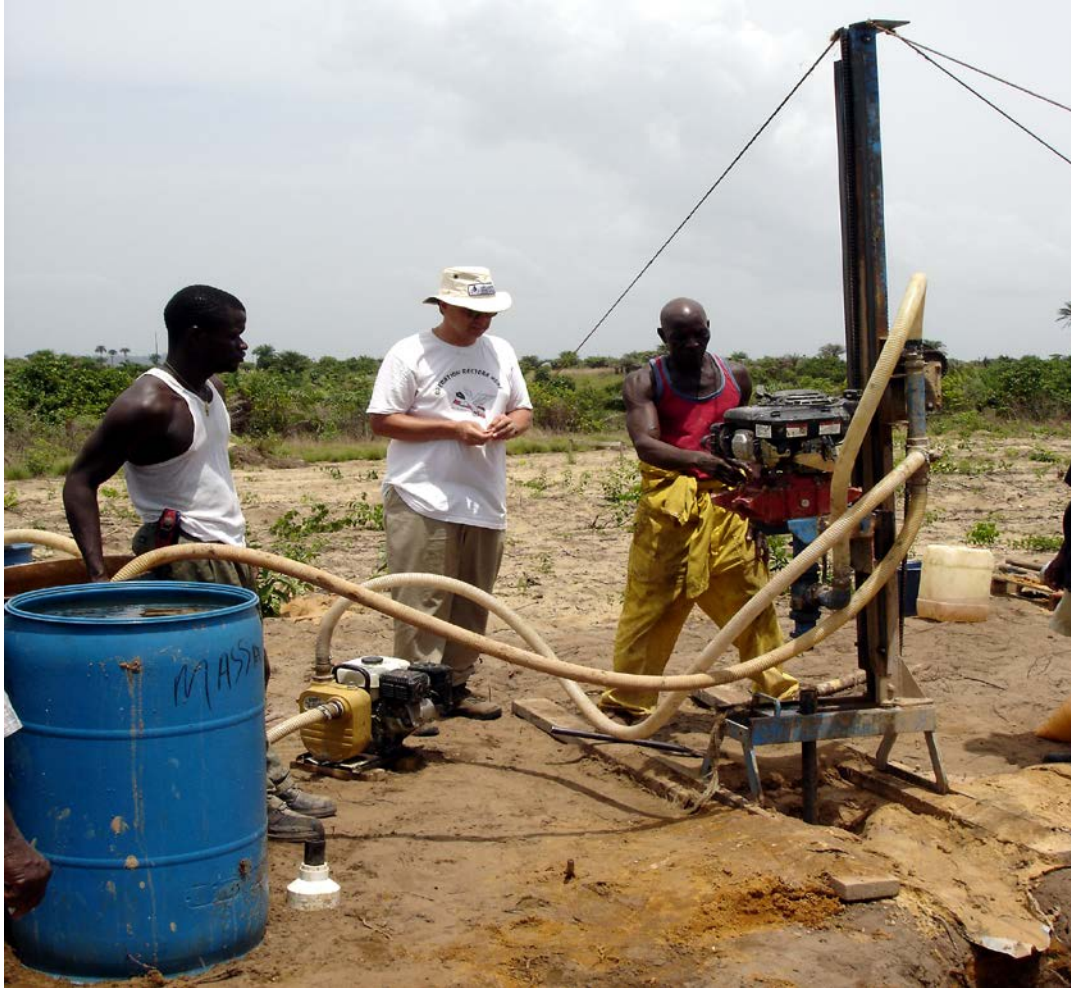
Jim Gehrels, founder of Lifewater Canada, trains new workers in Liberia how to safely drill water wells with an LS100 from Lone Star Drills. A strong component of Lifewater's program is local involvement at every level.
