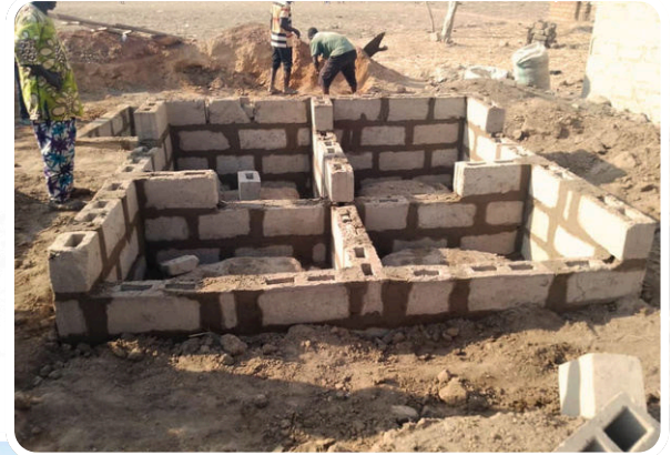
New Community washroom in Agyaragu- Koro
